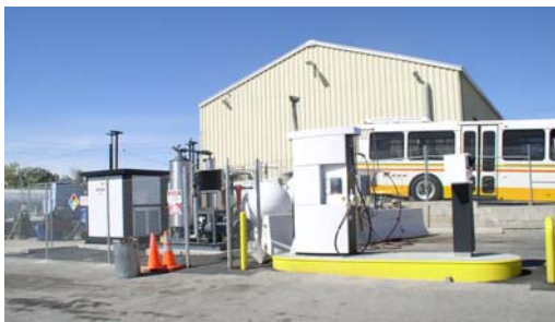
Figure 1: Completed CNG Station
