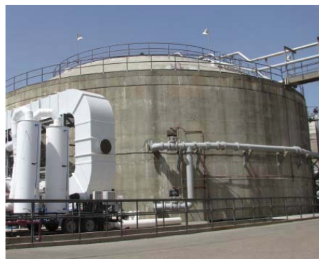
Figure 5: OCSW Wastewater Digester Tank
