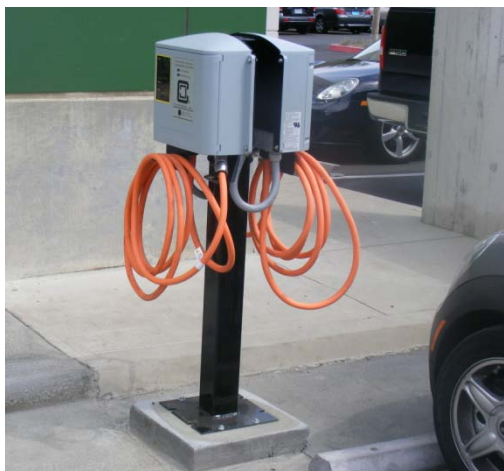
Figure 7: EV Charger Installed at SCAQMD HQs
