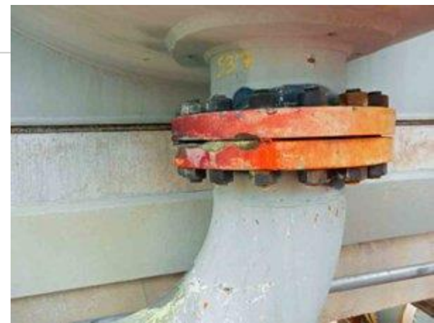
Flange that failed in Corpus Christi Release (21 tons)
