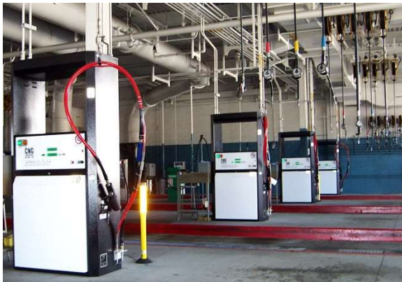
Figure 1: Single-Hose CNG Dispensers
