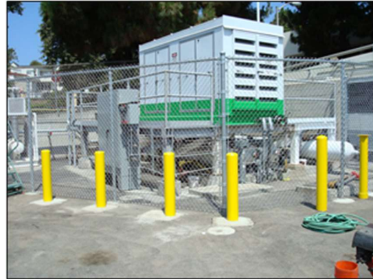
Figure 1: Compressor with Catwalk
