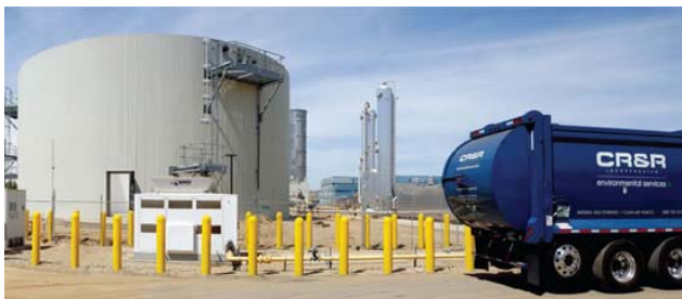
Figure 16: CR&R's Anaerobic Digester
