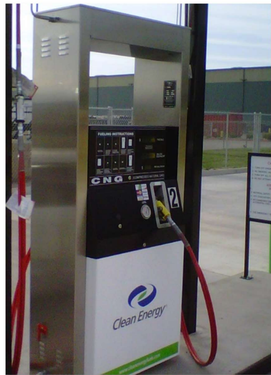
Figure 2: CNG Dispenser installed at Agua Mansa LNG Station
