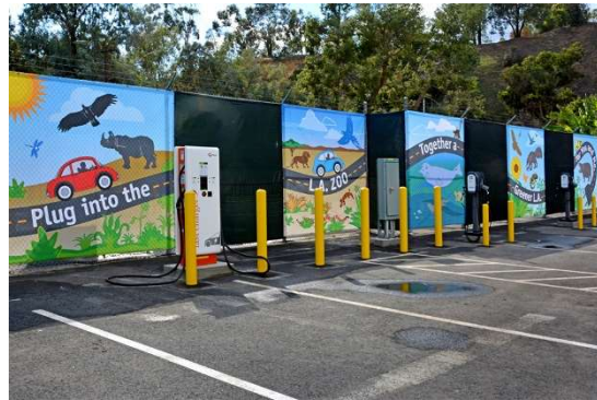
Figure 1: Los Angeles Zoo, DC Fast Charger and Level 2 EVSE (electric vehicle supply equipment)
