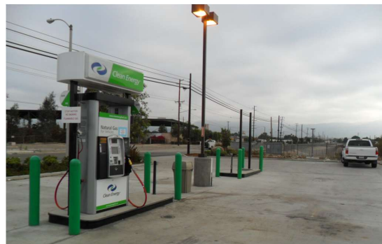
Figure 2: Foothill Transit CNG Station
