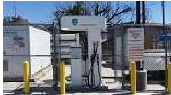
Figure 1: Burbank H2 Station
