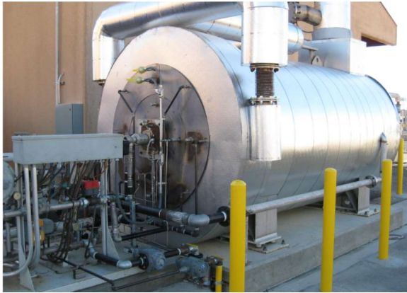
Figure 1: TVRWRF Noxtech® Reactor
