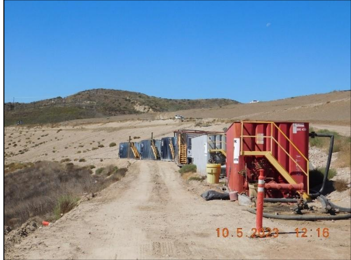
Figure 6 - Baker Tanks for temporary leachate storage.
